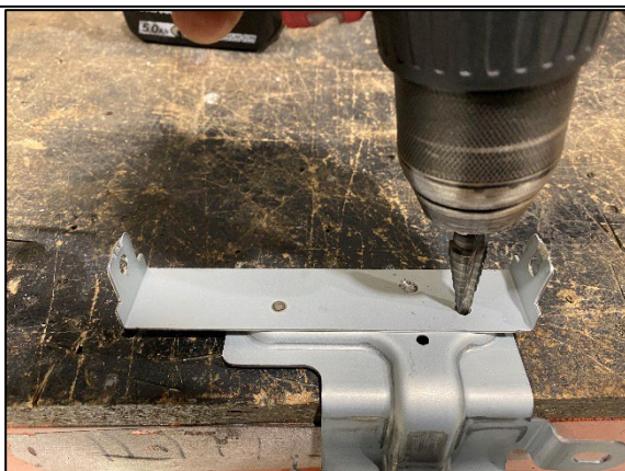
STEP 2.3 USING A 5MM DRILL BIT, DRILL OUT THE SPOT WELDS TO SEPARATE THE TWO SECTIONS OF THE BRACKET.
